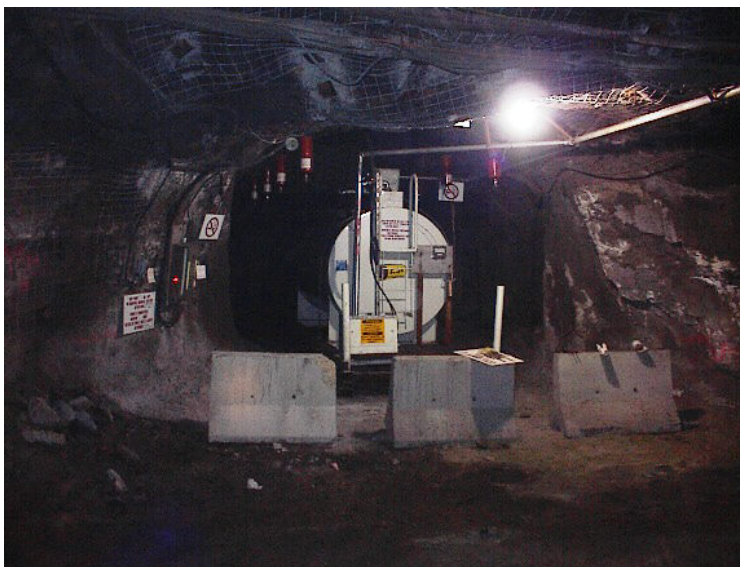
Figure 22 - Blended Fuel Storage at 1000 Level
